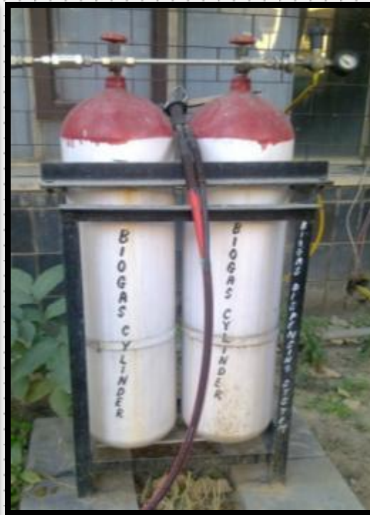
Two cylinder cascade for bottling of upgraded biogas
